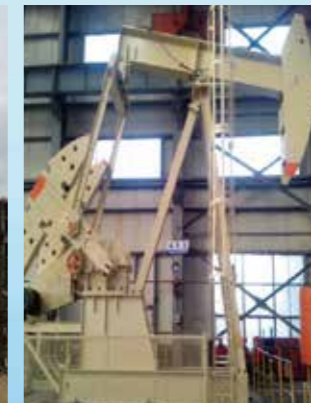
Beam Pumping Unit
