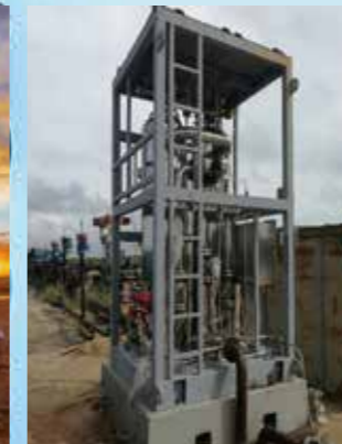
Double-separator Metering Device
