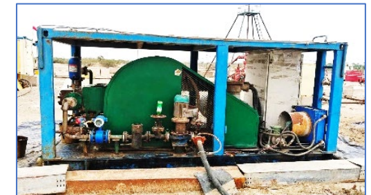
Pressurized Water Injection Equipment
